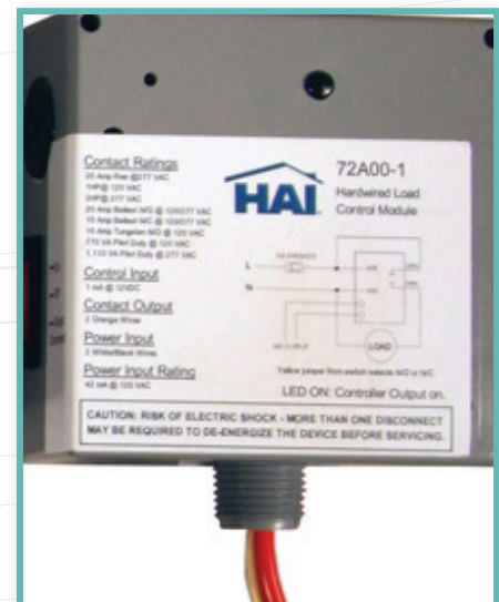
With Smart Grid, load control switches like the one pictured here can be set to lock out loads during expensive, peak power periods.
